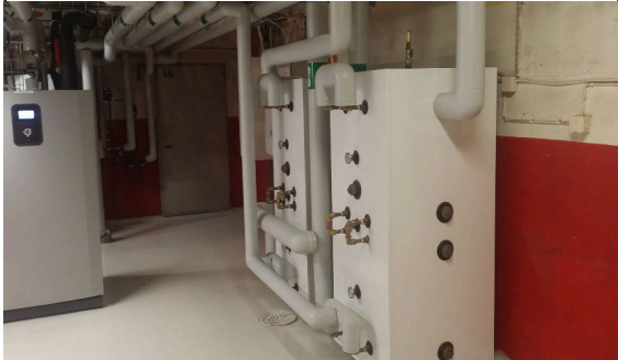
Plantroom 2 x Water tank 750 l.
